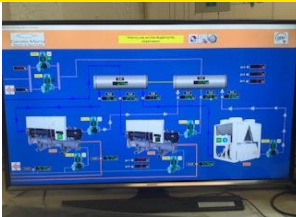
Clima & Heating operational recorders
