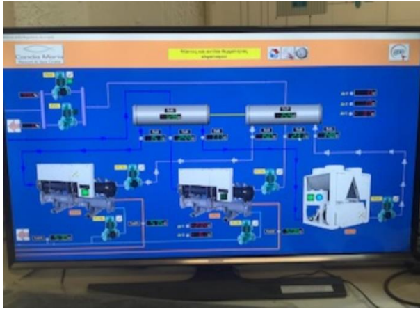
Clima & Heating operational recorders
